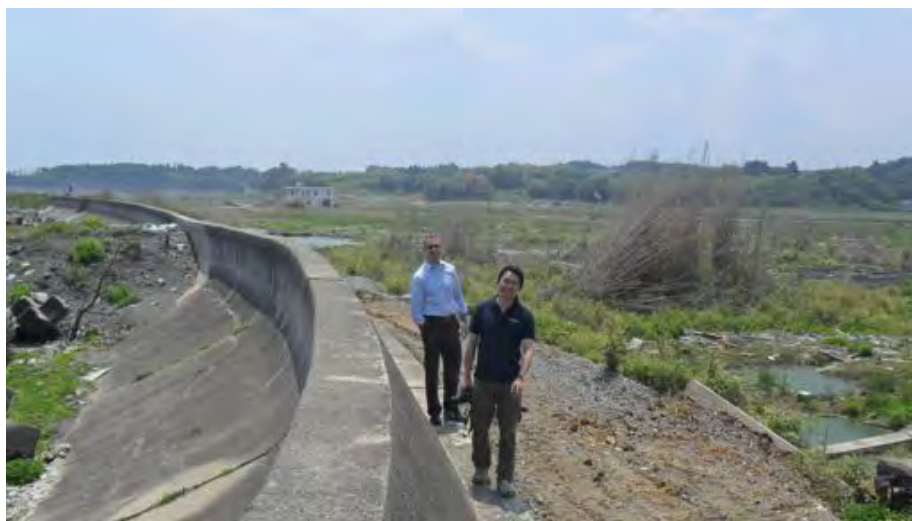
The tsunami wall that was unable to contain last year's tsunami.
